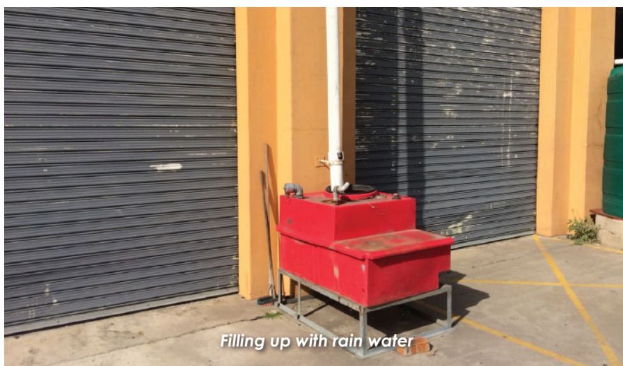
Water storage tanks with capacities of 5 000 litres or more were purchased and installed at every fire station in the city
